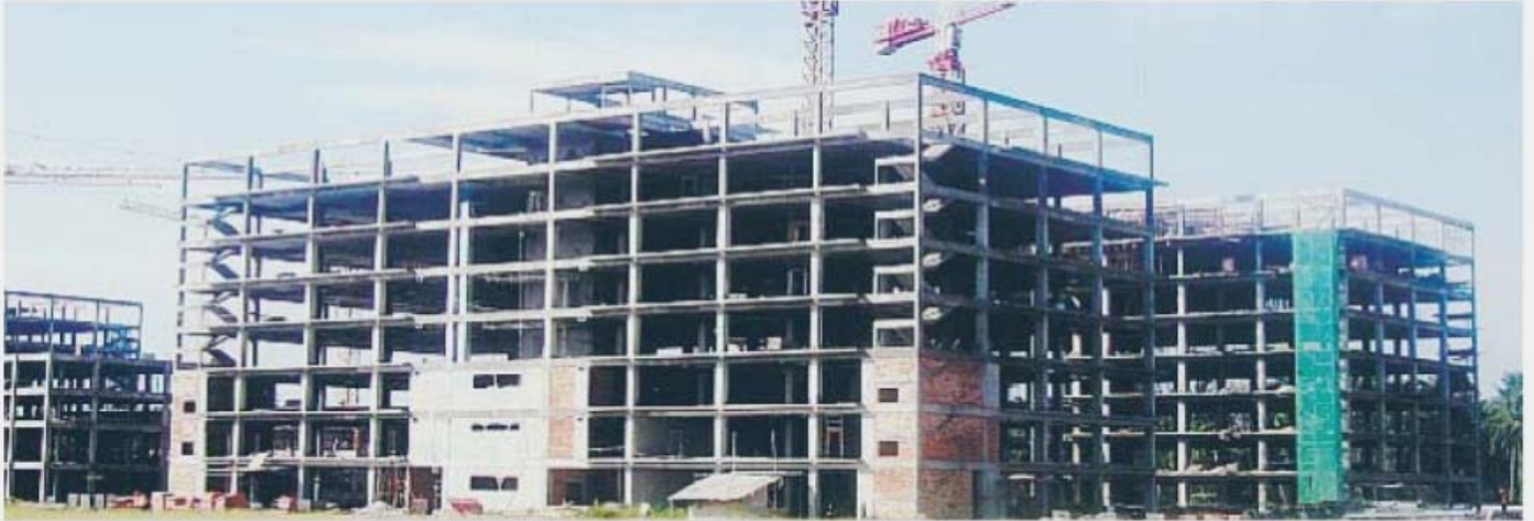
One of the buildings being constructed at the Port Klang Free Zone
